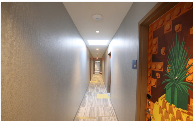
UniFi AC Pro AP mounted on a hallway ceiling
