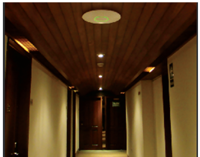
UniFi Access Point installed in hallway for guest rooms
